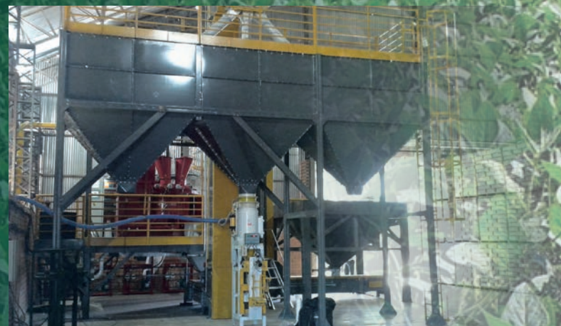
Complete Installation of CC250 including intake and packing line
