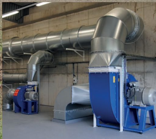
Aspiration with recirculation system
