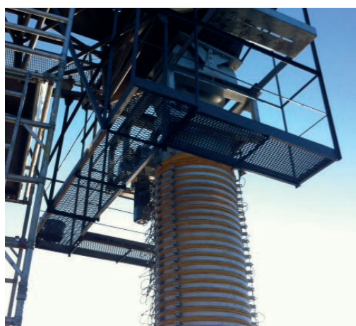
Loading chute installed in the Port of Liepaja at conveyor showing the cardan joint
